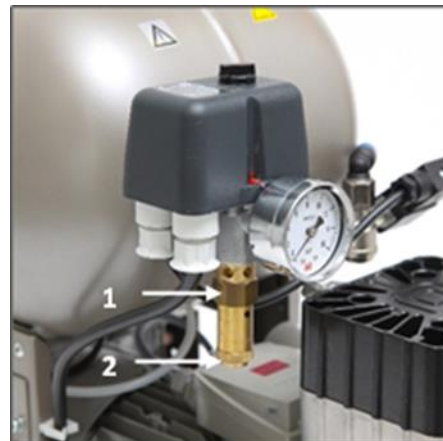
Fig. 7: Check of safety valve
